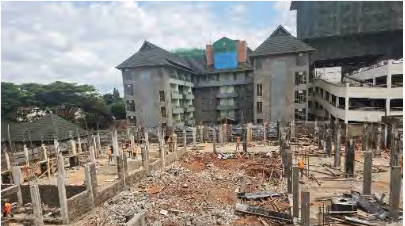
A cross section view of the ongoing reconstruction work at the reconstruction and modernization of the Desmond Tutu Conference Centre.
